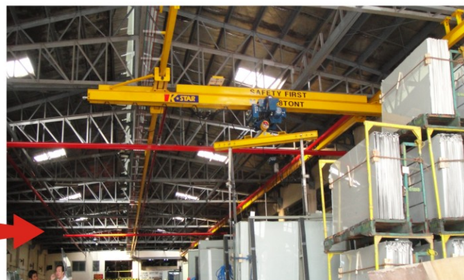
Suspension Crane (After)
