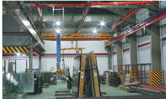
Overhead crane with LRS system
