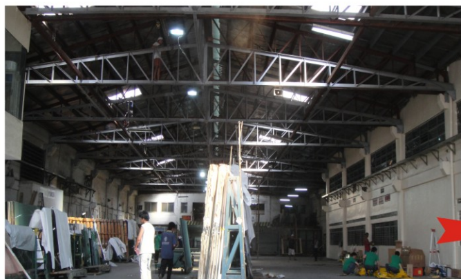
Suspension Crane (Before)
