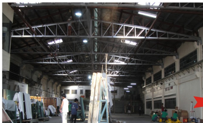
Suspension Crane (Before)
