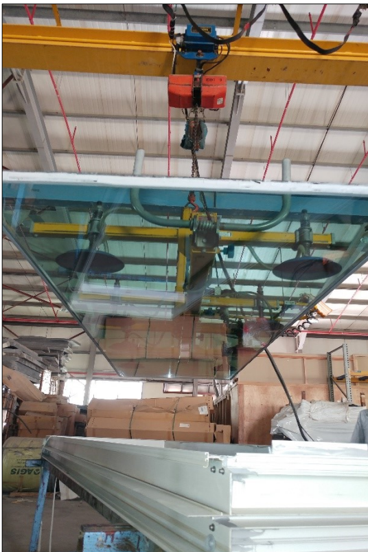
Figure 28: Glass pane completely removed from frame.
