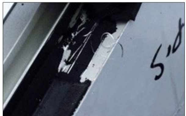
Figure 32: Example with black SG joint - Adhesion failure.
